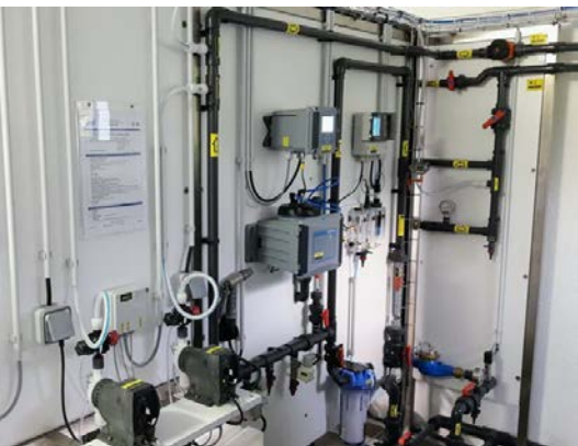
Figure 3: view of the control, sampling and monitoring
