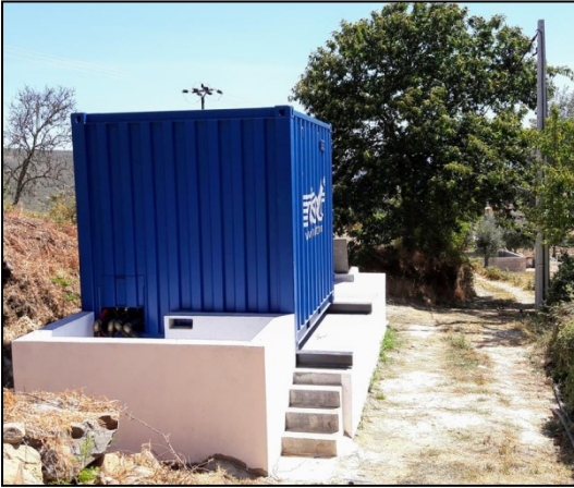
Figure 1: Treatment water conditioning assemble on a 10' sea container
